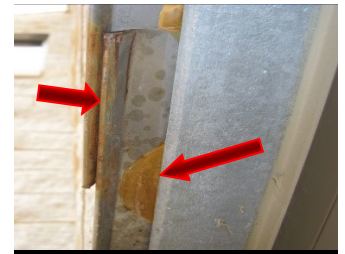
Always protect metals from cleaning...Including Stainless Steel (Drip Edges)... use blue tape
