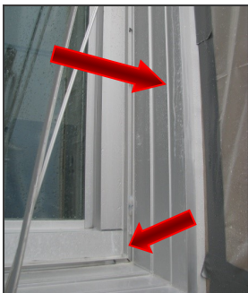
Aluminum frame permanently stained by masonry cleaning.
